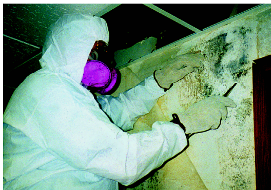
Photo 7: Remediation worker with limited PPE
