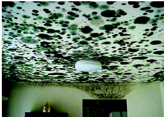
Photo 2: Extensive mold contamination of ceiling and walls
